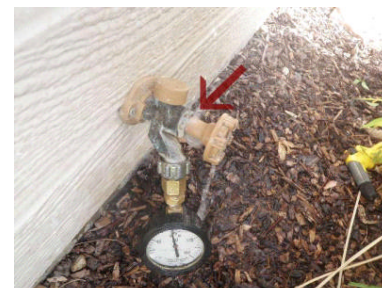
Front Hose Faucet Leaks at Handle
