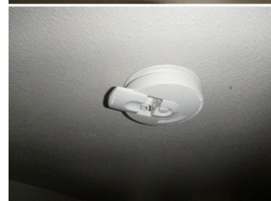
Smoke Detectors Need Backup Batteries
